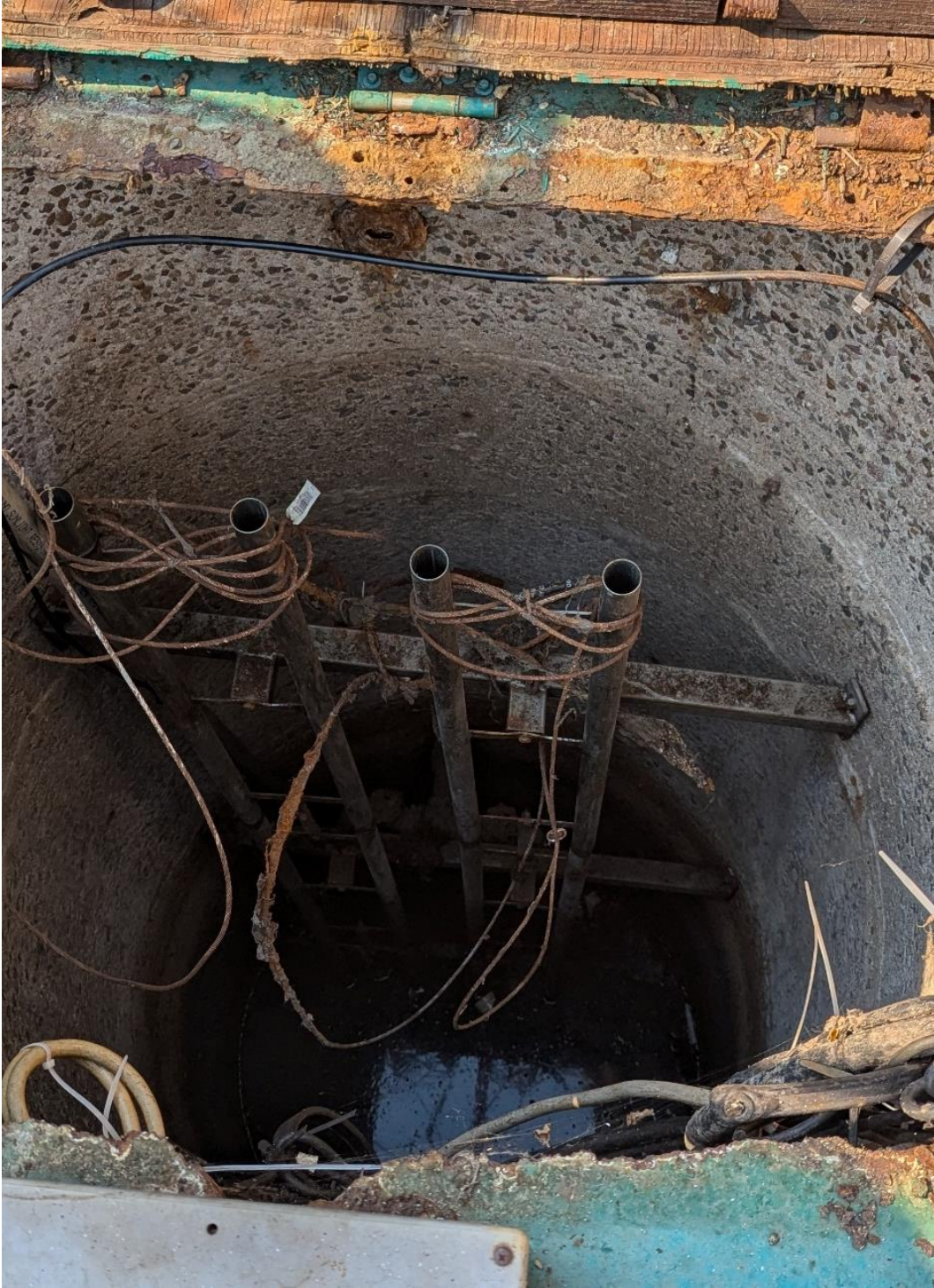
Figure 5 Oak Tree Lift Station Wet Well and Cover Condition
