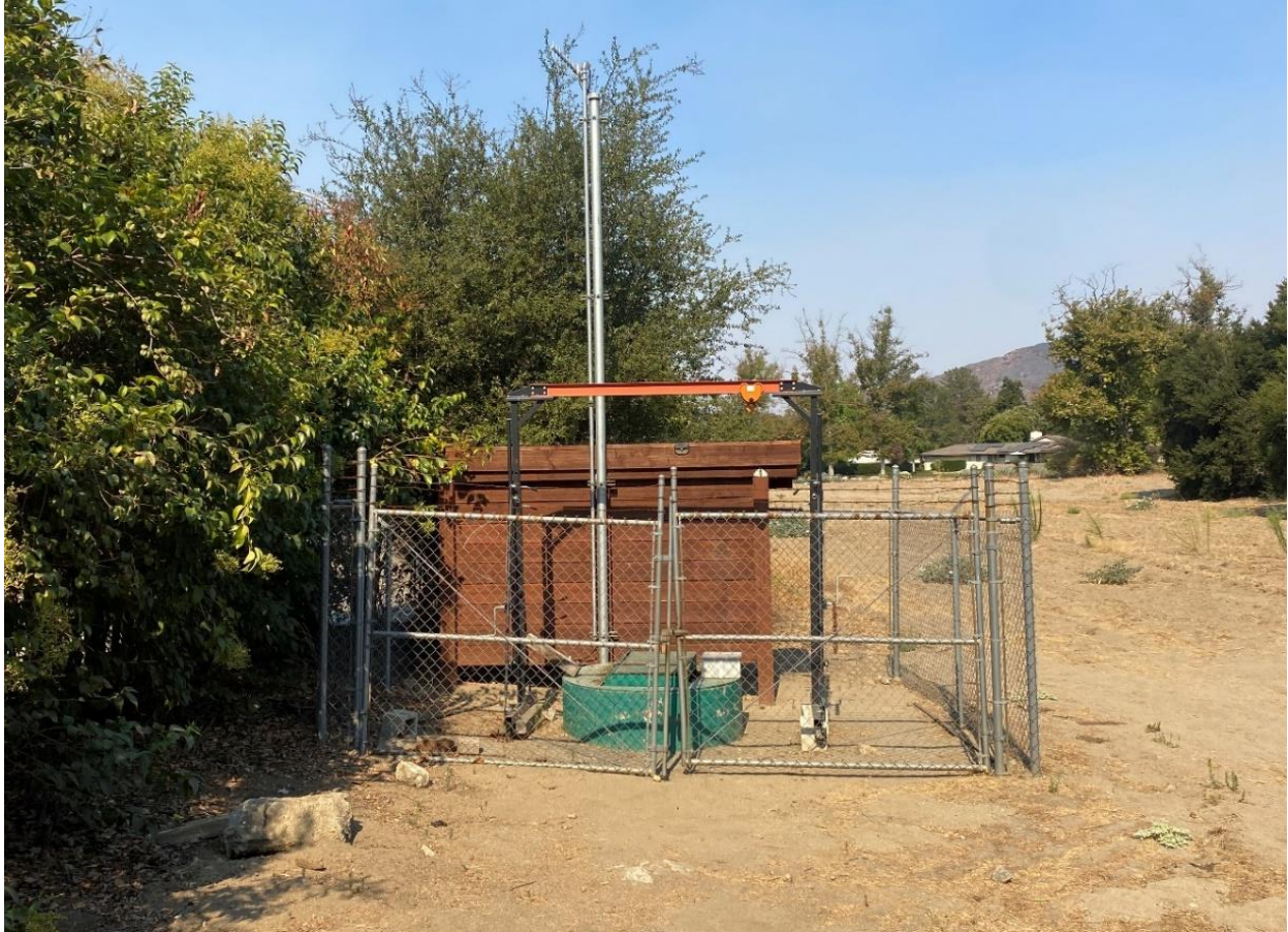
Figure 3 Oak Tree Lift Station
