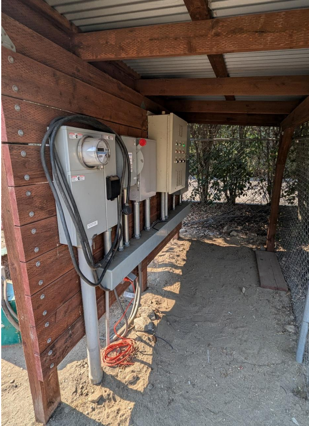
Figure 4 Oak Tree Lift Station Electrical Equipment
